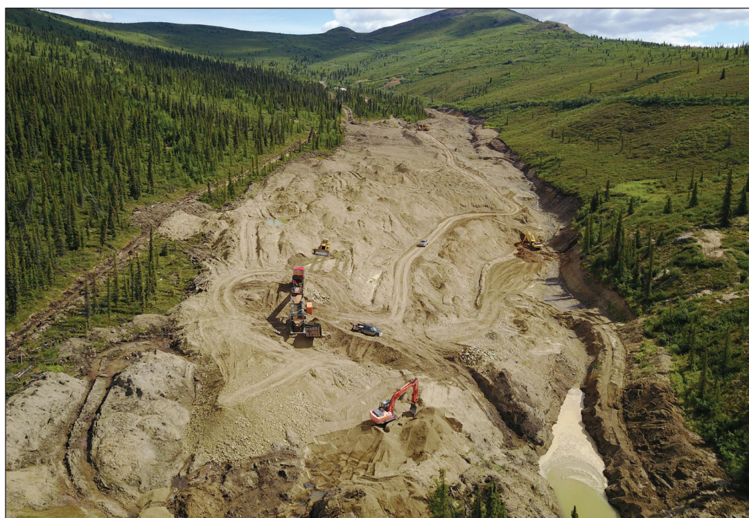
Figure 16. Aerial view looking upstream Webber Creek at Capital Gold Mining Corp.'s operation this season.
