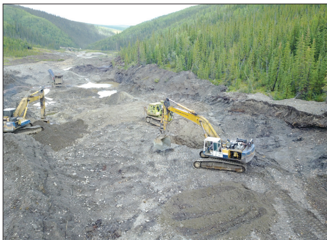
Figure 9. Chrysos Mining processing a low-level, right limit bench deposit on Bruin Creek.
