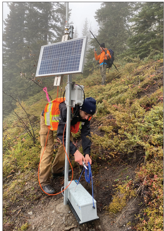
Figure 7. BGC Engineering staff installing an extensometer on the Moosehide Slide in September, 2022.
