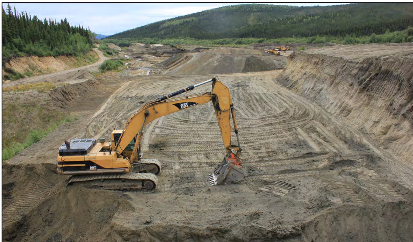
T.D. Oilfield Services Ltd. 2014 cut below Laskey Lake, looking downstream.
