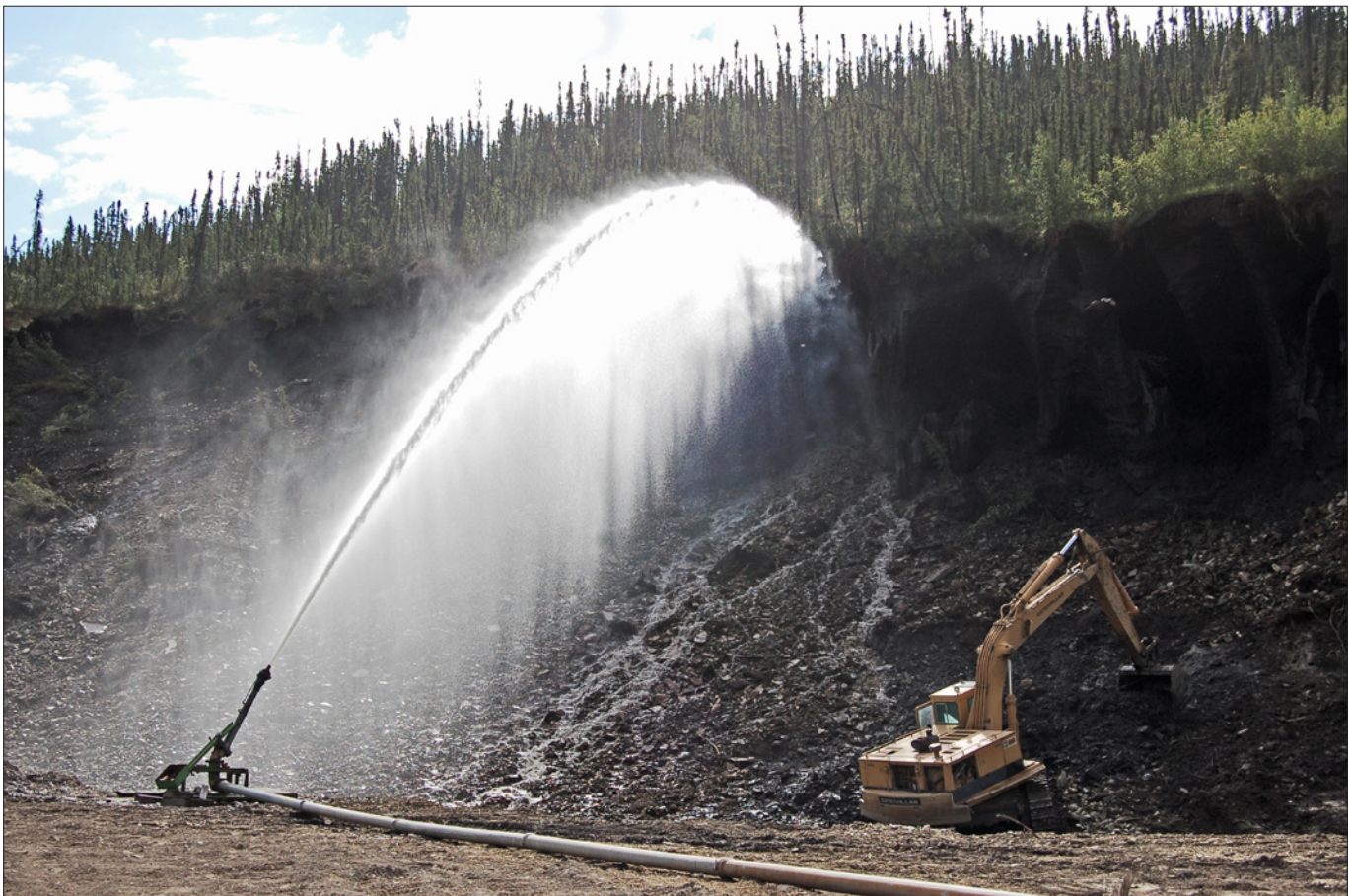
Hydraulic and mechanical stripping on the left limit of Hunker, Henry Gulch Placers, 2006.
