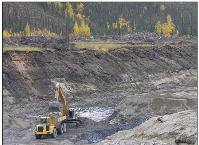
T.D. Oilfield Services pit on the left limit of Klondike River at the mouth of Hunker Creek, 2003.
