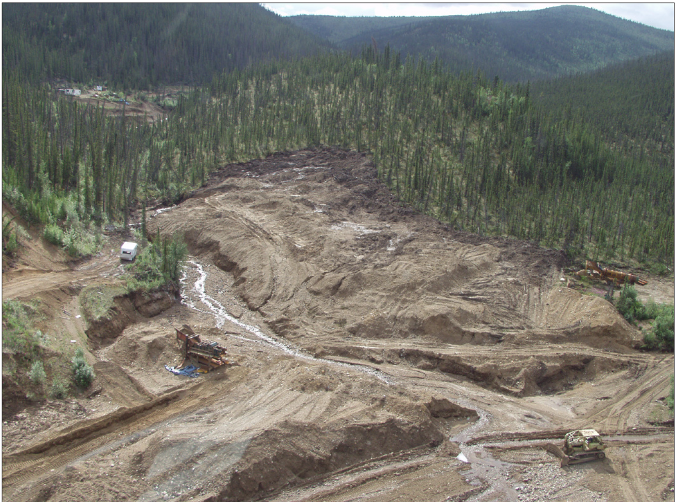
Hank Fehr's bulldozer and two sluice plants on Mechanic Creek, 2003. Wes Darling's operation can be seen in the upper left background.
