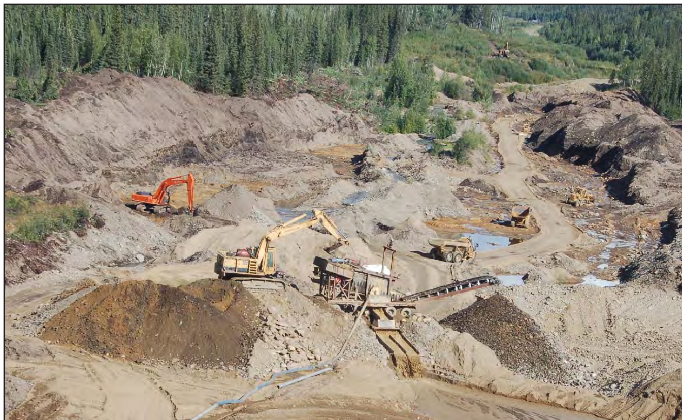
View of the wash plant and cut of Fell-Hawk Placers mining operation on Kirkman Creek in 2008.
