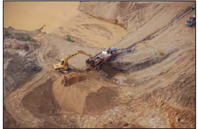
Spring Cove Enterprises wash plant at their upper West Victoria Creek operation in 2007.
