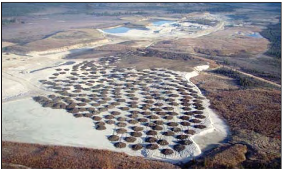
Ross Mining Ltd. dumped topsoil for spreading on this sloped and contoured previously mined site.
