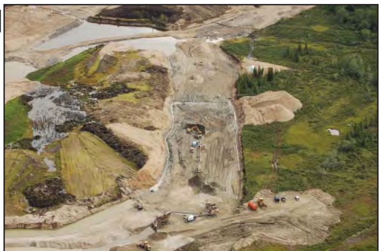
Aerial view of Gimlex Enterprises Ltd's mining cut on Indian River in 2008.
