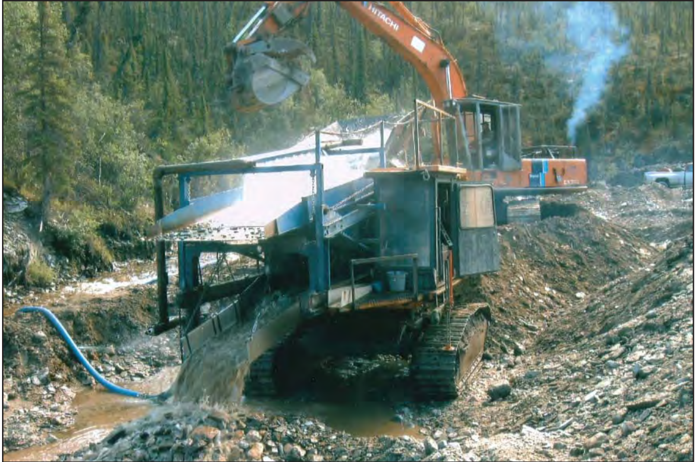
Daniel Jones' wash plant on Moose Creek was mounted on an excavator undercarriage for ease of portability.
