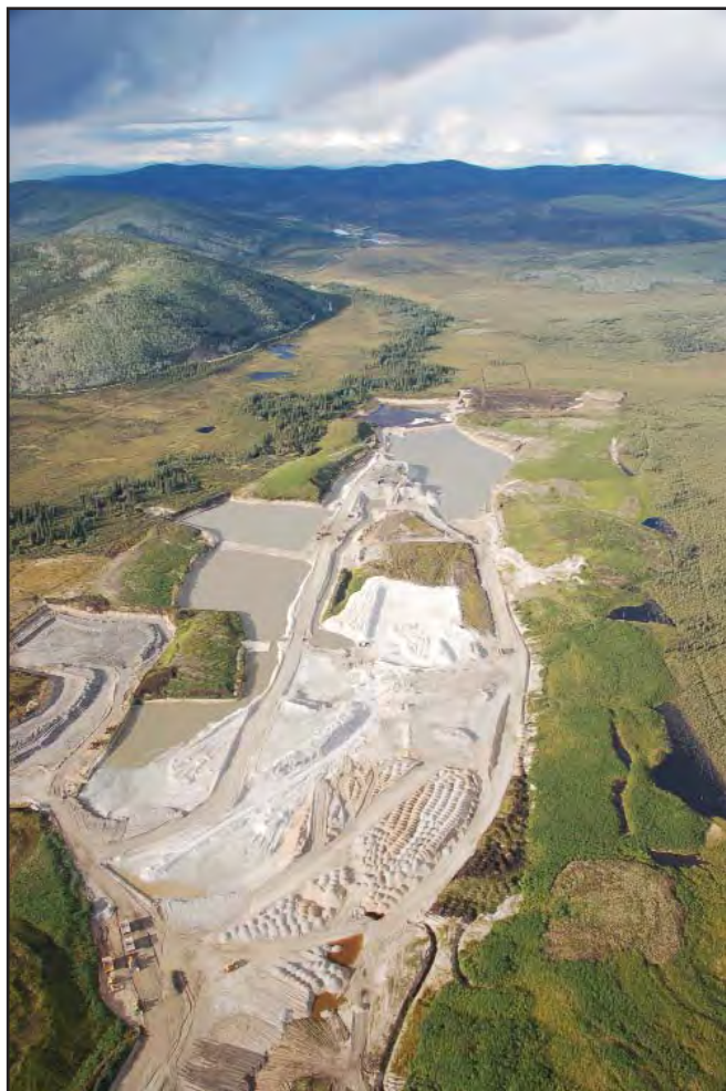
Ross Mining Ltd. on Dominion Creek was the largest operating placer mine in Yukon in 2008.
