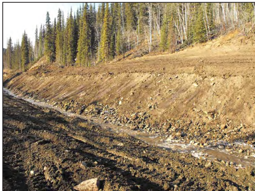
Re-sloped and contoured overburden piles along the creek allow for safe passage of migrating wildlife.
