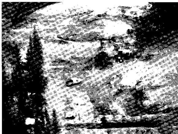
Sluicing in progress on Robert Stirling's property located on a bar deposit close to the McQuesten airstrip.
